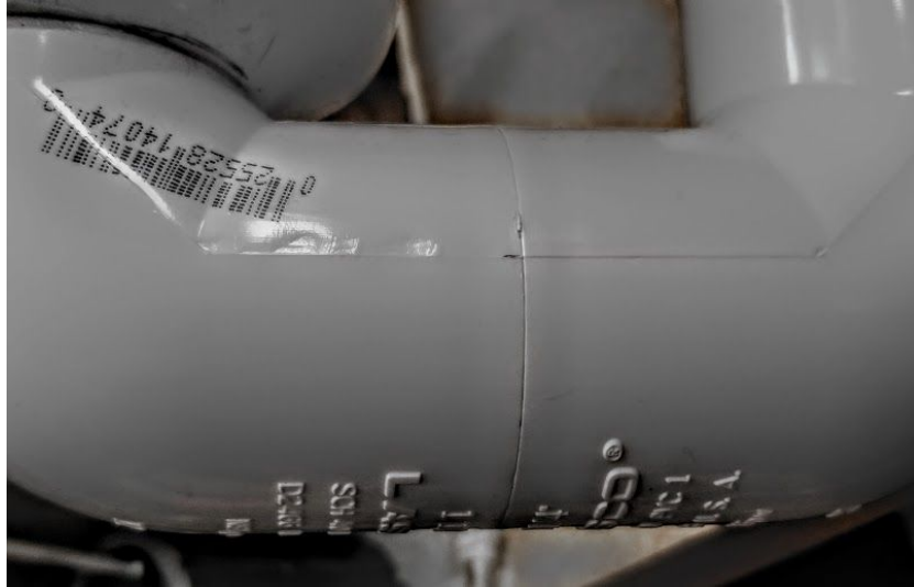
“U” Elbow Seams Lined Up
