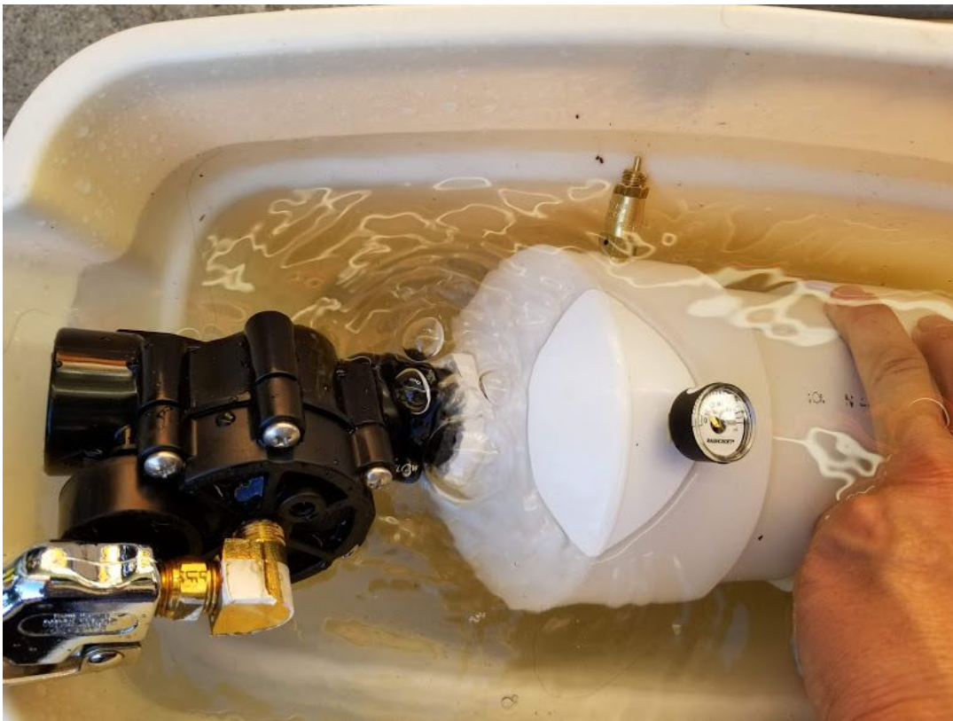
Leaking in the Main Valve Threads
