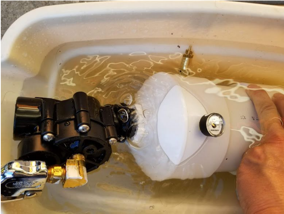
Leaking in the Main Valve Threads
