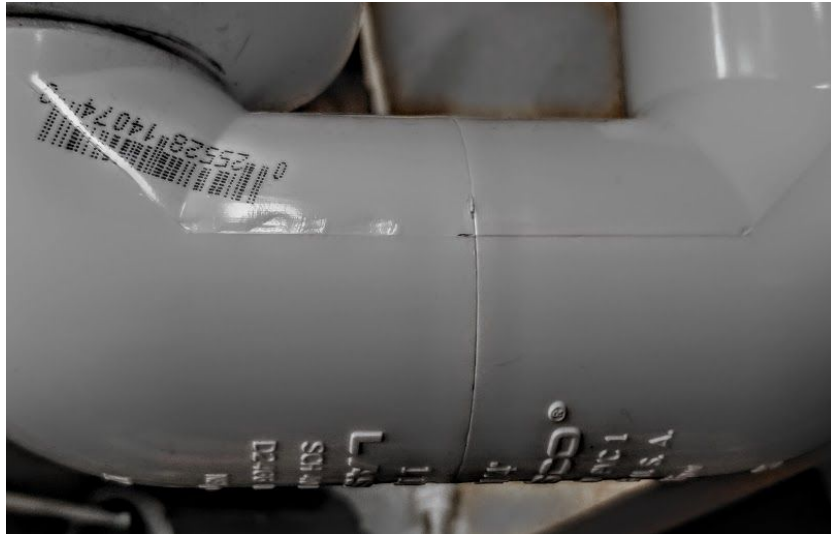
“U” Elbow Seams Lined Up
